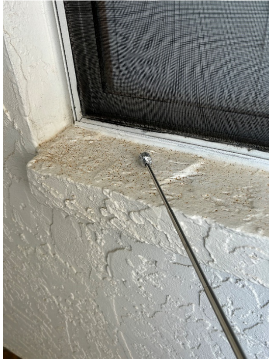
Minor Isolated Spall Identified on Sixth Floor Walkway, Unit 602
