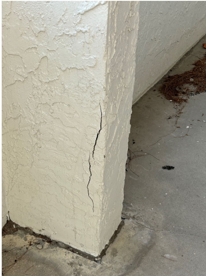
Visual Crack Forming at Column of North Parking Garage
