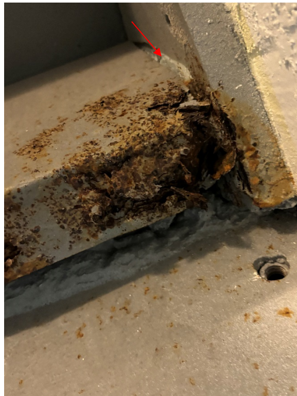
Observed Rusting and Minor Section Loss for Identified Concrete Filled Steel Pan
