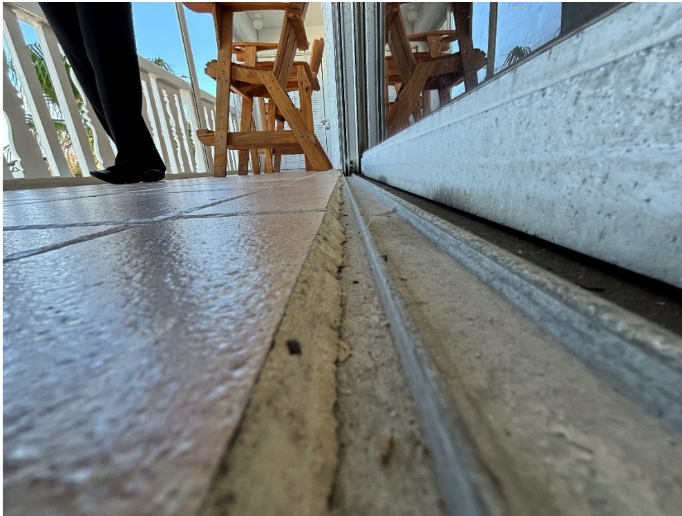
Sliding Glass Door Threshold Below Tile Finish Unit 502
