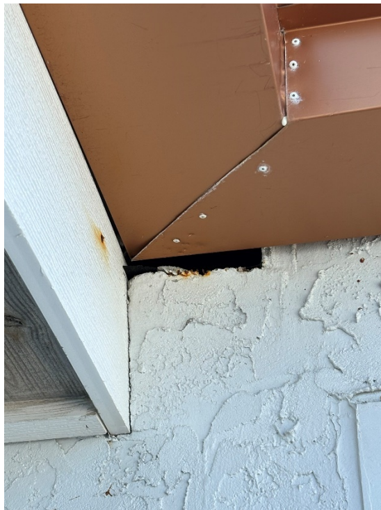
Void at Unit 704 Balcony Wall
