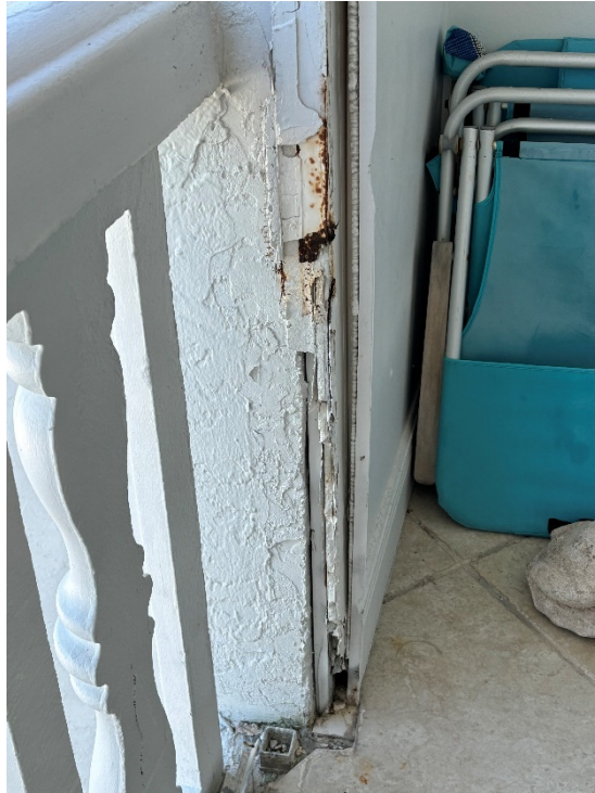
Additional Damage at Balcony Unit 701
