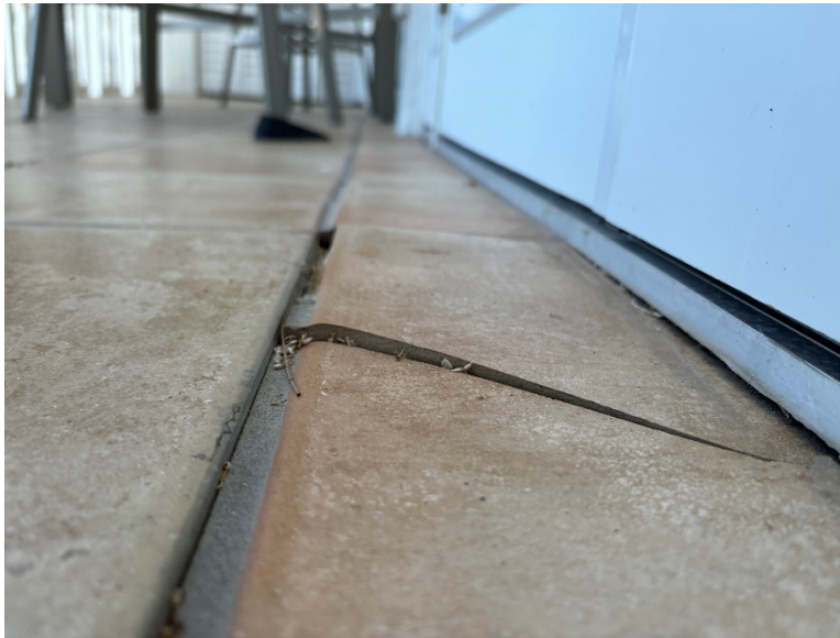
Damaged Tile at Balcony Door Threshold Unit 402
