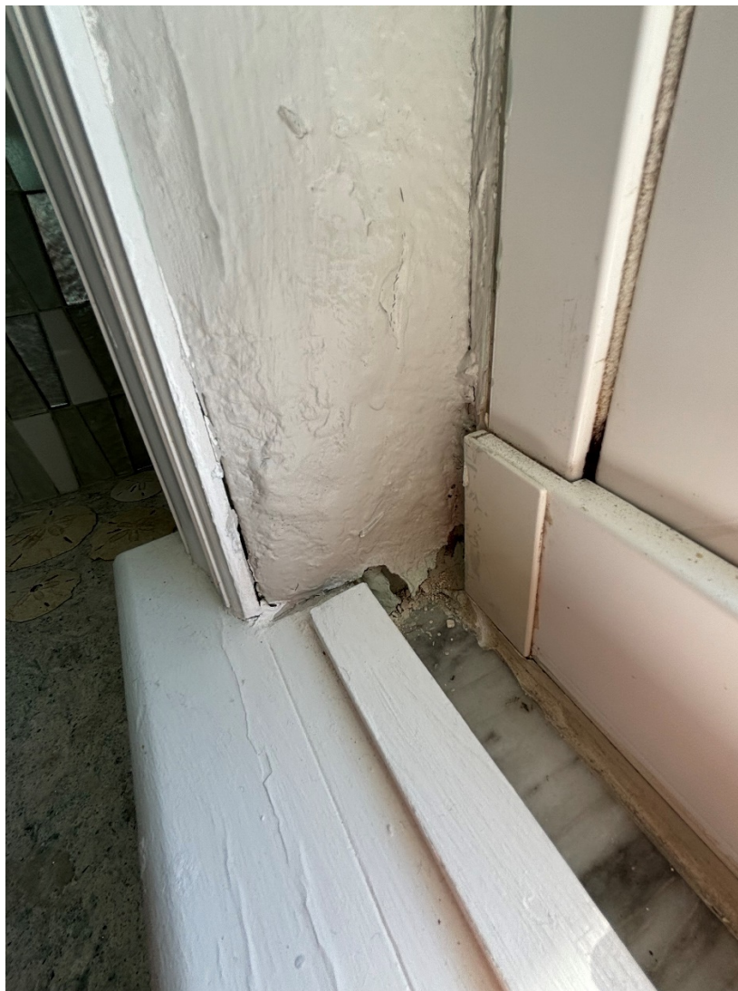
Water Damage at Kitchen Window Unit 301
