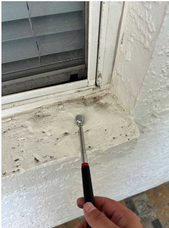
Minor Isolated Spall Identified on Third Floor Walkway, Unit 302
