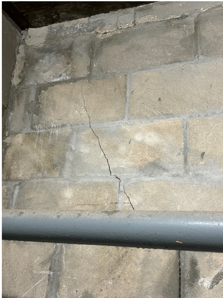
Crack Formed in Concrete Masonry Wall of Elevator Room
