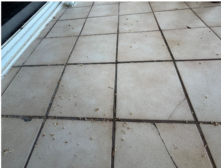
Area of Tenting Tile/ Hollow at Balcony Unit 203
