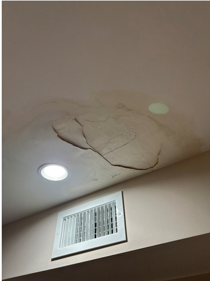
Water Damage at Ceiling of Unit 704
