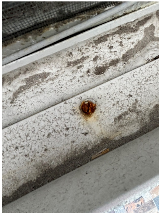
Rusting Fasteners at Identified Exterior Window Sills with Shutters
