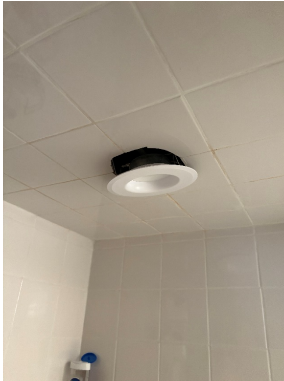
Unit Owners in Unit 603 Stated Water Leaks Occurring in Bathroom
