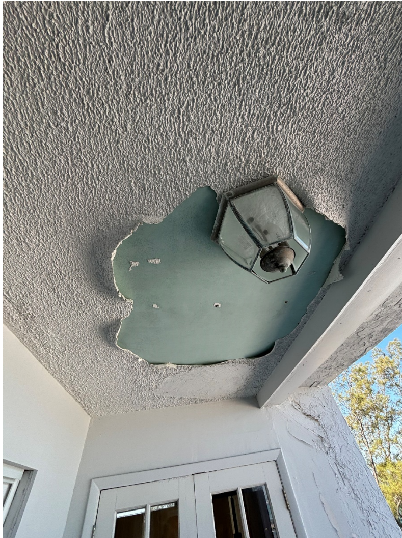
Damaged Ceiling Finish Unit 701
