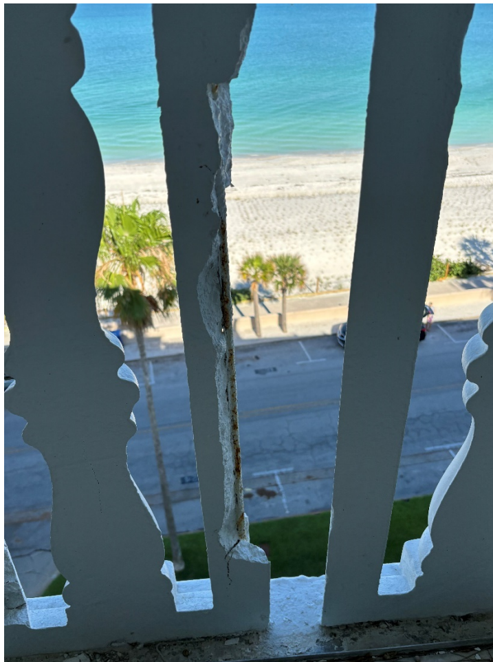
Exposed Reinforcement at Concrete Guardrail Unit 701
