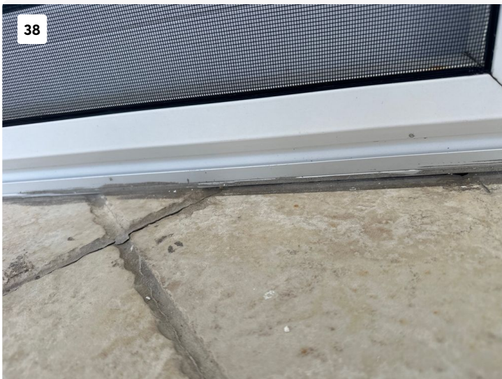
Cracks in tile and deterioration of sealant along base of slider.
