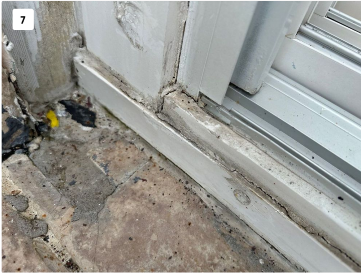
7 Heavy use of sealant along base of sliding glass door with widespread deterioration of sealant and separations present.
