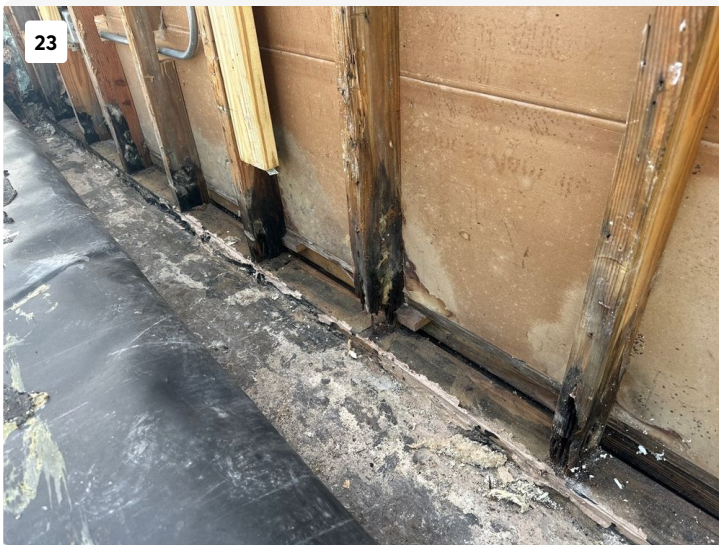
23 Widespread deterioration of base of vertical studs on wall of Unit 701. Portions appeared to have previous repairs on studs.
