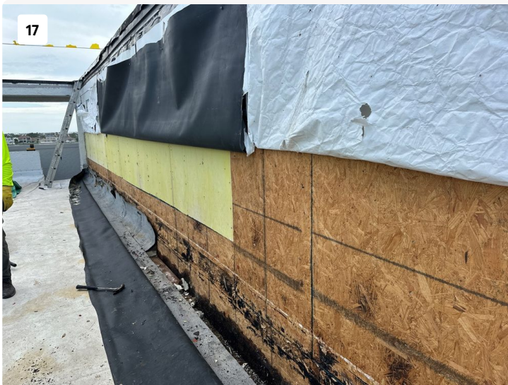
Base of OSB sheathing on 701 wall adjacent to lower roof found to have widespread deterioration along the base.
