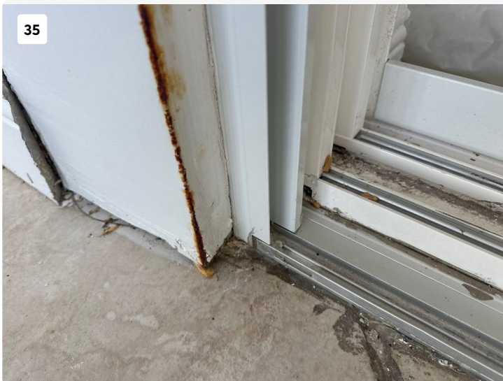
Base of slider and base of wall unsealed.
