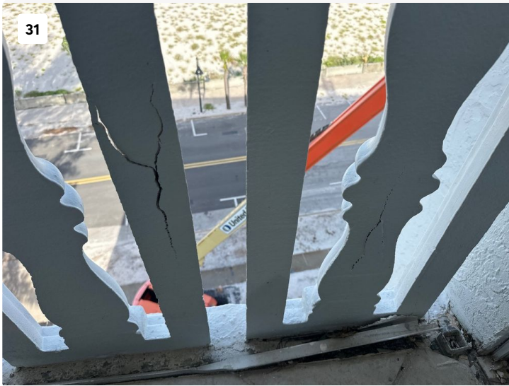
Widespread spalling of rails on balcony on 701.
