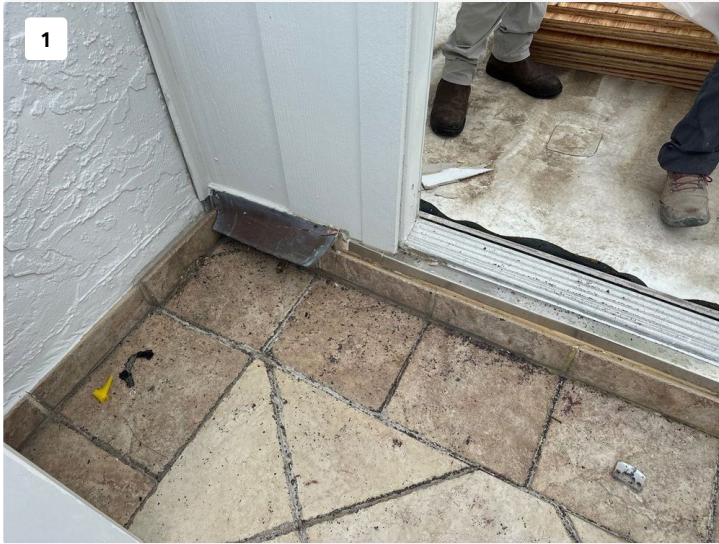
Large balcony of Unit 701 base of wall. Vertical tile has separations present along base of existing opening.
