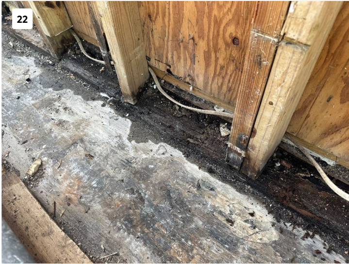
22 Water observed to continuously leach out from under interior tile of Unit 701 into low roof area.
