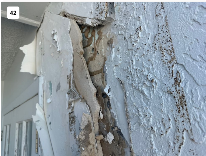
Wall of balcony had widespread deterioration present. Found to have drywall glued to exterior wall and was crumbling.
