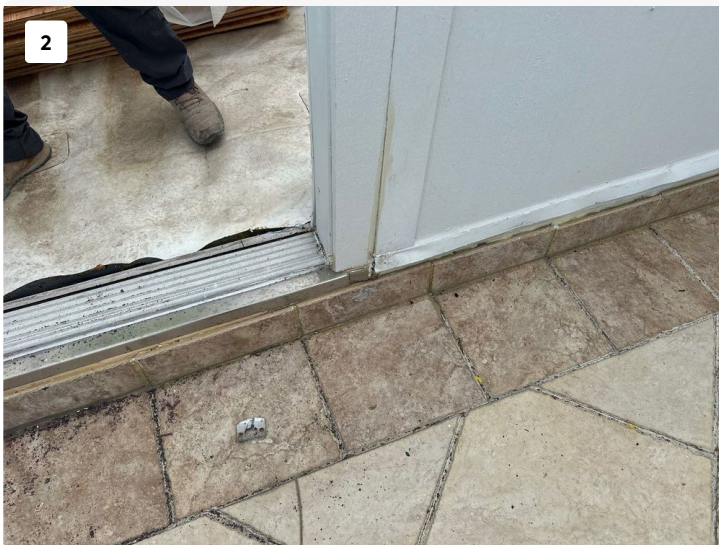
Large balcony of Unit 701 base of wall. Vertical tile has separations present along base of existing opening.
