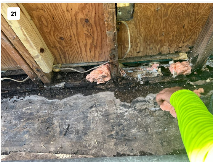
21 Water observed to continuously leach out from under interior tile of Unit 701 into low roof area.
