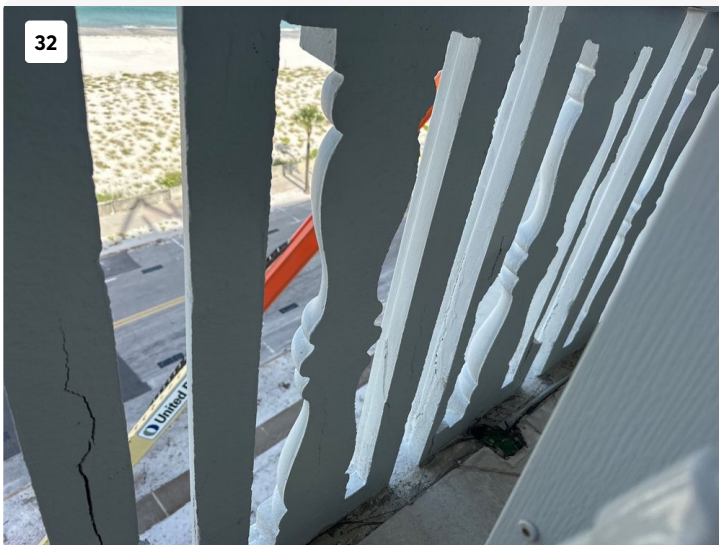
Widespread spalling of rails on balcony on 701.
