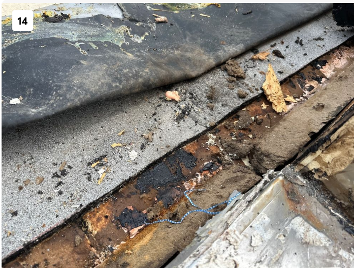
Insulation board on lower roof area on side of 701 found to have widespread areas of trapped moisture.
