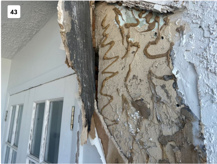
Wall of balcony had widespread deterioration present. Found to have drywall glued to exterior wall and was crumbling.
