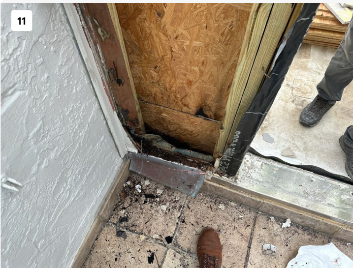
Apparent previous framing repairs along side of door as well as deterioration of oriented strand board (OSB) sheathing under wall finishes.
