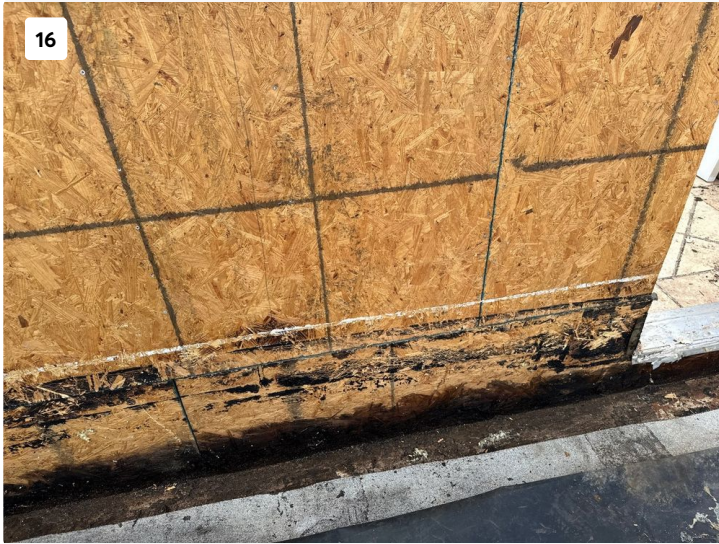
Base of OSB sheathing on 701 wall adjacent to lower roof found to have widespread deterioration along the base.
