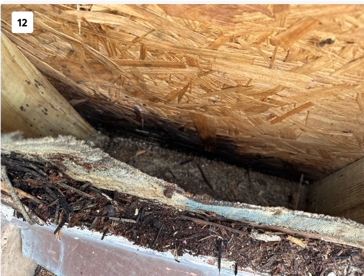
Apparent previous framing repairs along side of door as well as deterioration of oriented strand board (OSB) sheathing under wall finishes.
