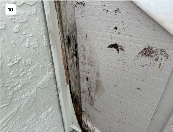
Upon removal of the hardieboard finish on sides of balcony door on 701 deterioration of covered T1-11 siding that was observed.
