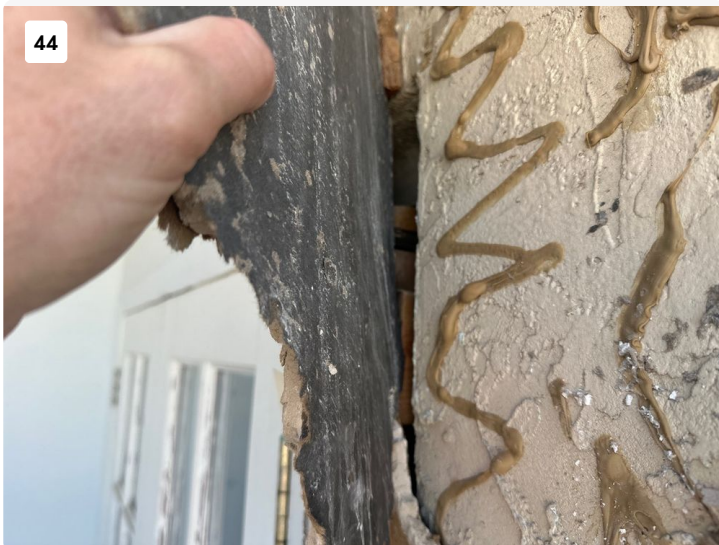
Opening for french door found to be open and not flashed.
