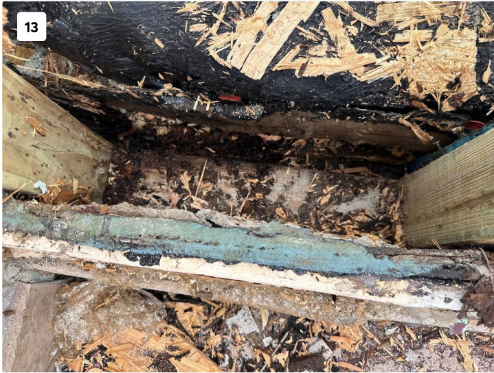
Apparent previous framing repairs along side of door as well as deterioration of oriented strand board (OSB) sheathing under wall finishes.
