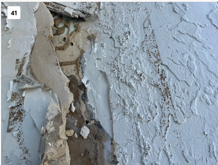
Wall of balcony had widespread deterioration present. Found to have drywall glued to exterior wall and was crumbling.
