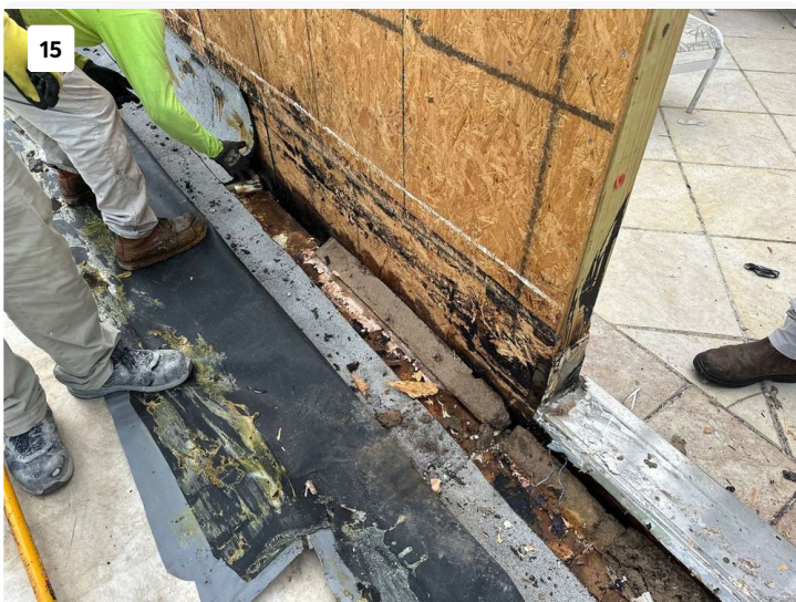
Insulation board on lower roof area on side of 701 found to have widespread areas of trapped moisture.
