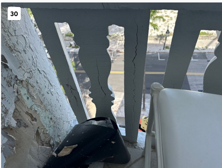
Widespread spalling of rails on balcony on 701.
