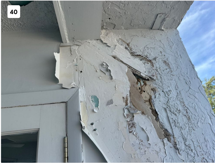
Wall of balcony had widespread deterioration present. Found to have drywall glued to exterior wall and was crumbling.
