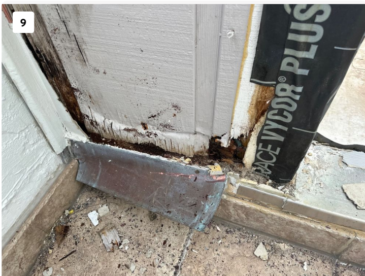
9 Upon removal of the hardieboard finish on sides of balcony door on 701 deterioration of covered T1-11 siding that was observed.
