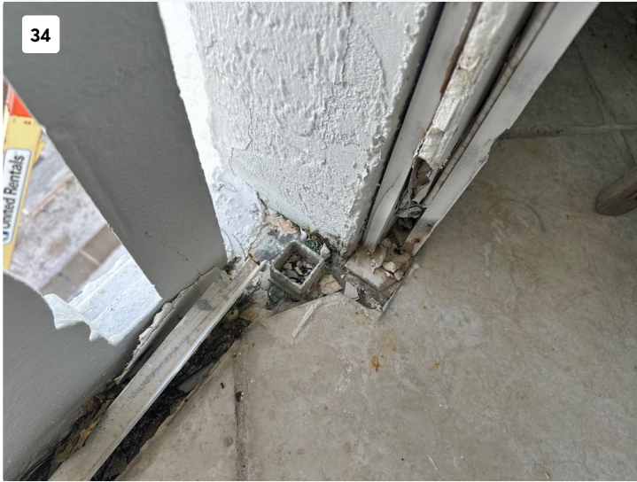
Multiple layers of drywall installed on the exterior walls of small balcony. Unsealed penetrations observed on balcony.
