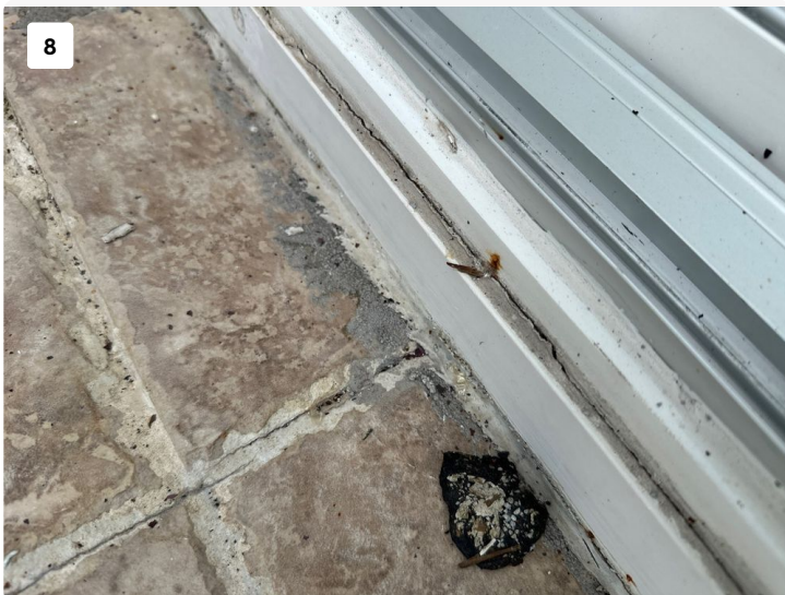
8 Heavy use of sealant along base of sliding glass door with widespread deterioration of sealant and separations present.
